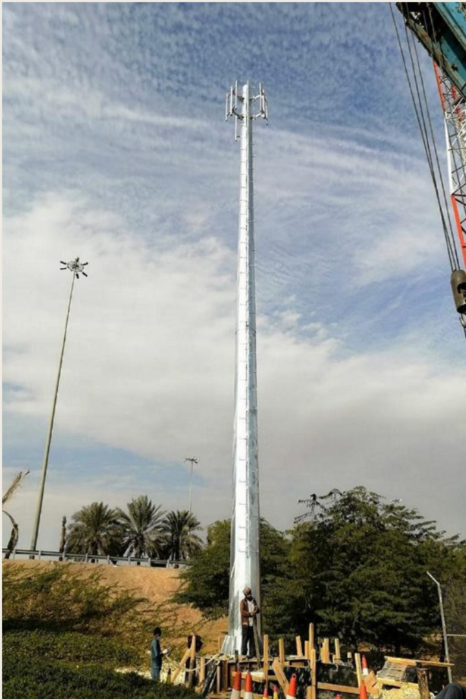
20m Radio Antenna Microwave Towers monopole
