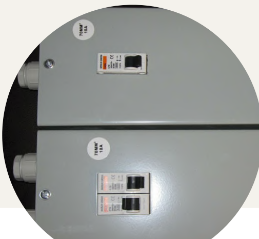
METAL FUSE BOX
